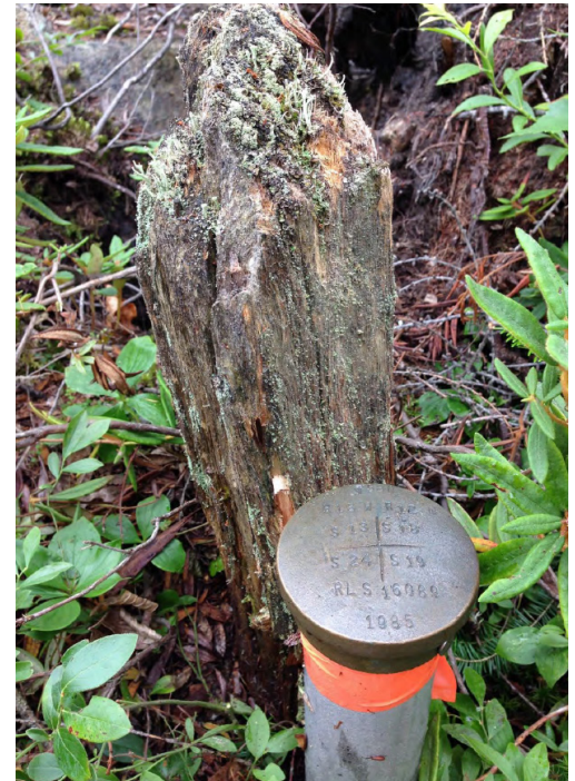
Brass-capped aluminum pipe monument (front) compared to previous wood post monument (back).
